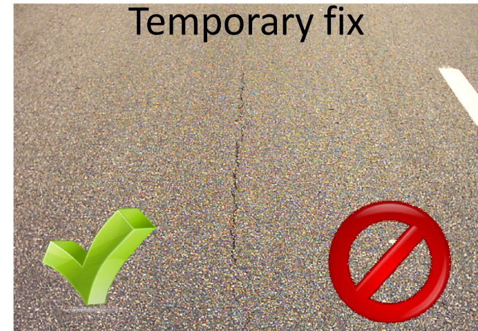
Longitudinal Cracking (wheelpath)
