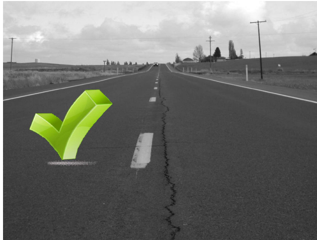
Longitudinal Cracking (not in wheelpath)
