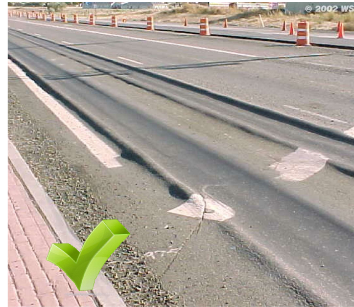
Rutting/Shoving (surficial/requires milling)
