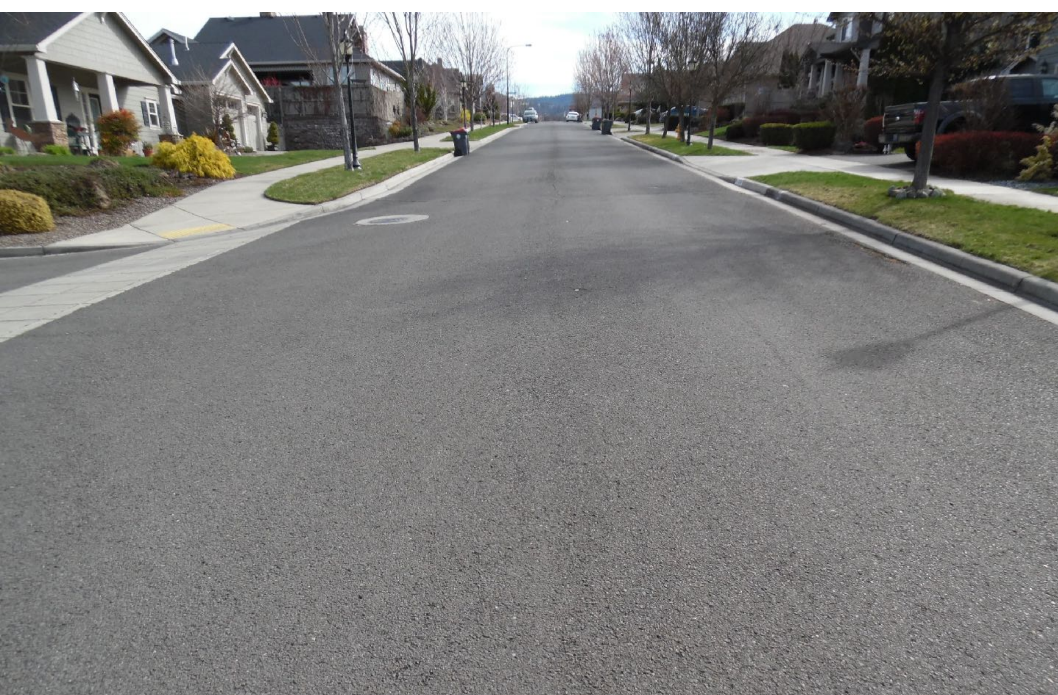
Fieldbrook Looking E. from W. of Link Dr. Paved 2003, Treated with RePlay 2010- PCI 83.7
