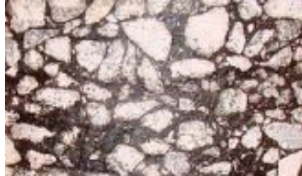
PCC Joint Cracking
