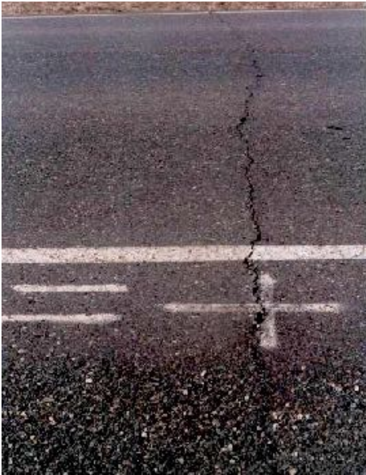
Crack #11 No GlasGrid
