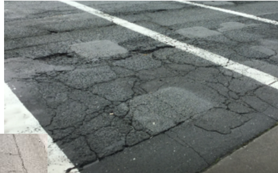
Delamination, Pop-outs, Trench Cut, Block Cracks
