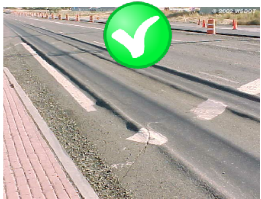
Surface Failure – Milling Required
