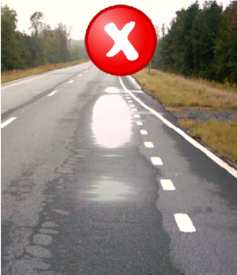
Severe Structural Failure
