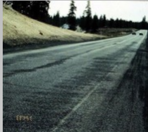
Snow Plow Damage
