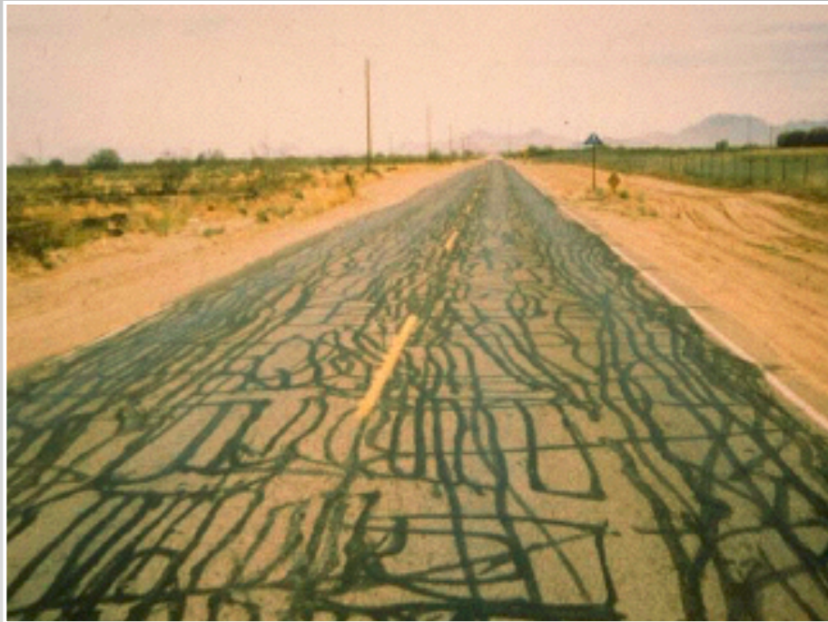
EXCESSIVE SEALANT Labor intensive
