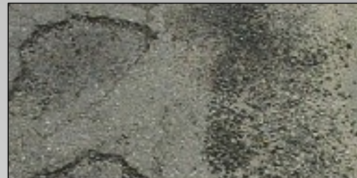
Weather, Traffic, Delamination
