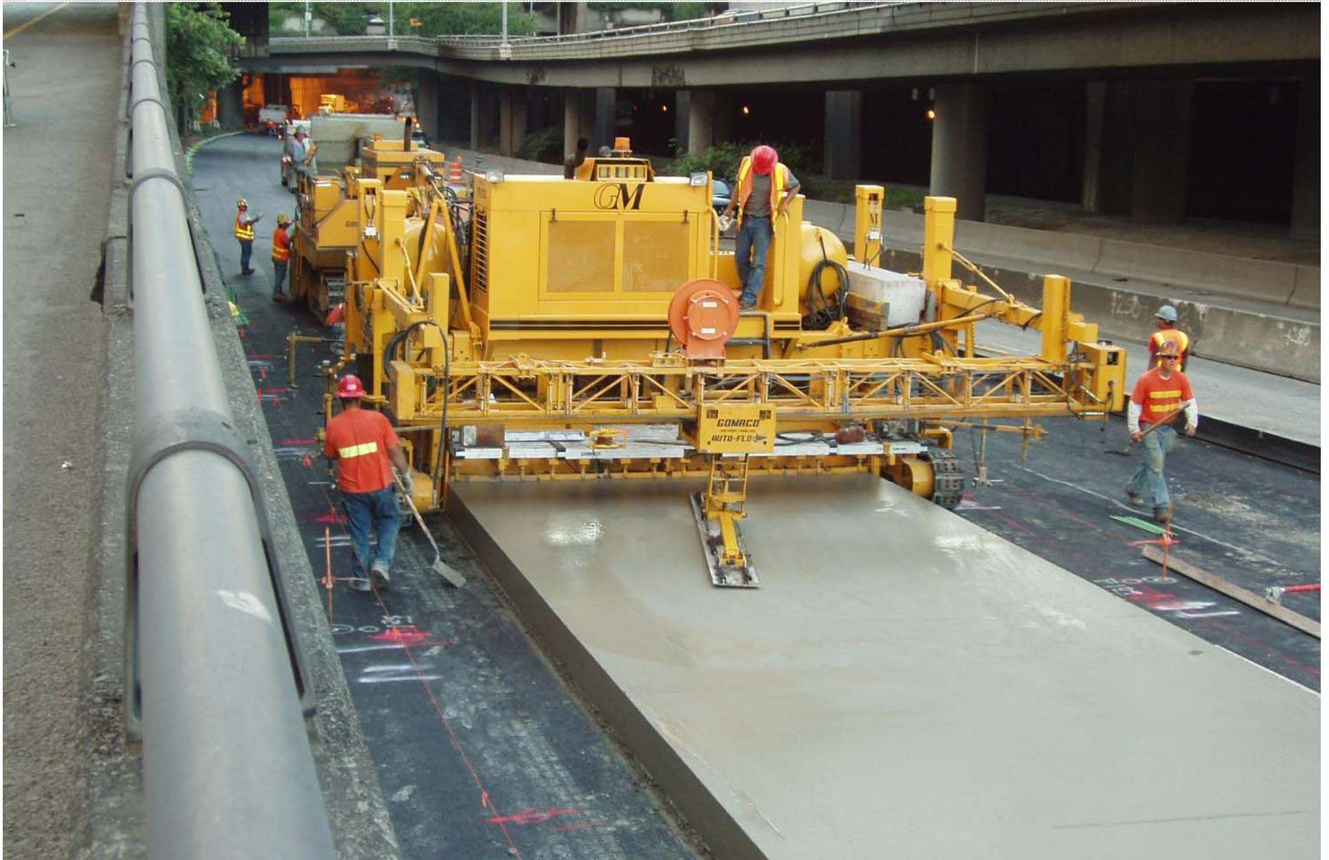
Paving 13 inches (330 mm) of jointed concrete pavement on I-5 in Seattle, Washington, United States
