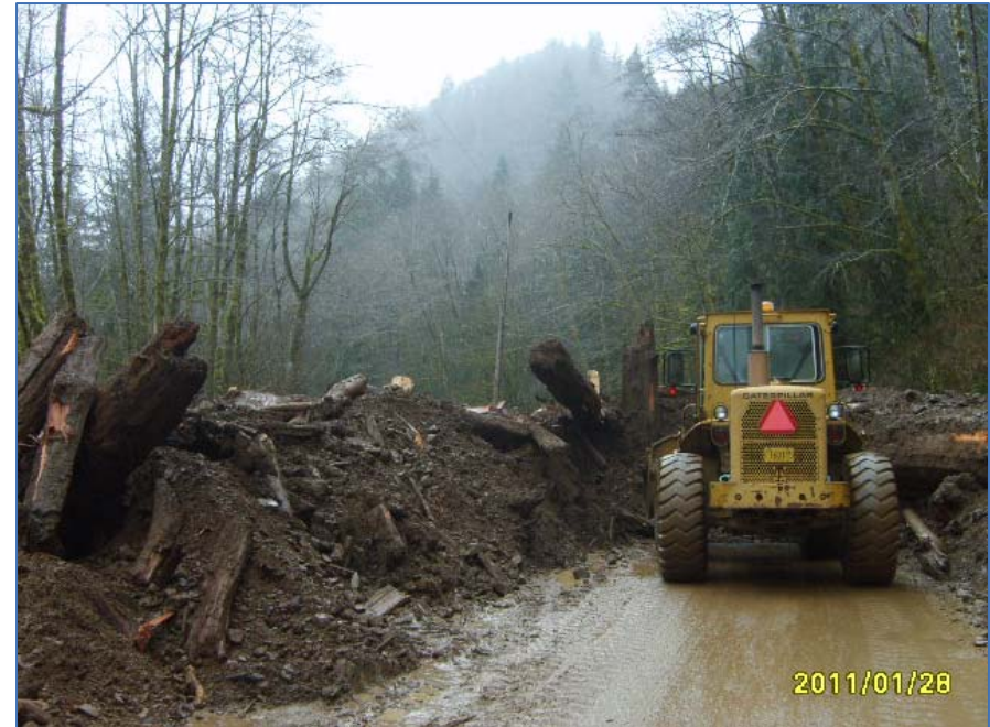
Foss Road, January 2011 Storm
