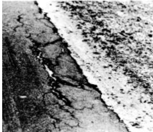
FIGURE A-5 Flexible pavement edge cracking (15).
