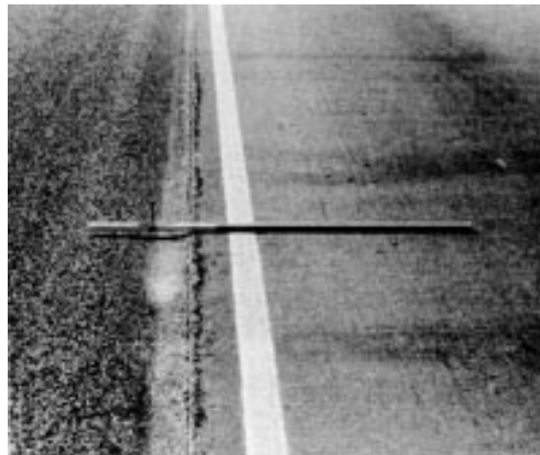
FIGURE A-6 Lane-shoulder dropoff (20).
