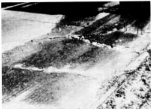
FIGURE A-9 Pumping of portland cement concrete pavement (20).
