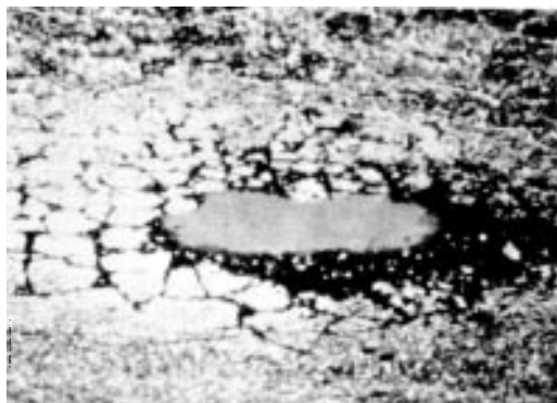
FIGURE A-3 Pothole (20).
